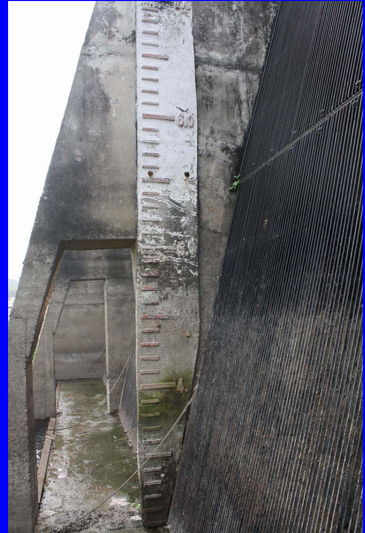
Bar screens on the outside
